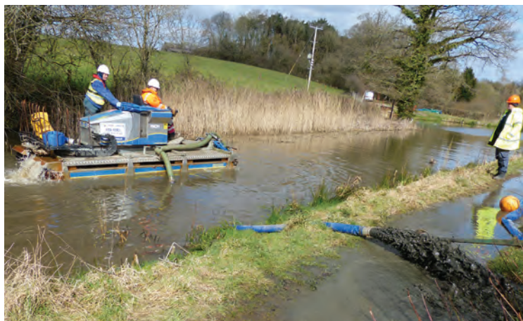
The amphibious machine at work pumping silt out of the canal near Loxwood.
