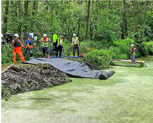
The SpeedyDam being put into action. It created a seal in a matter of hours. Water on the bridge side was pumped out to allow excavation for the diverted gas main.
