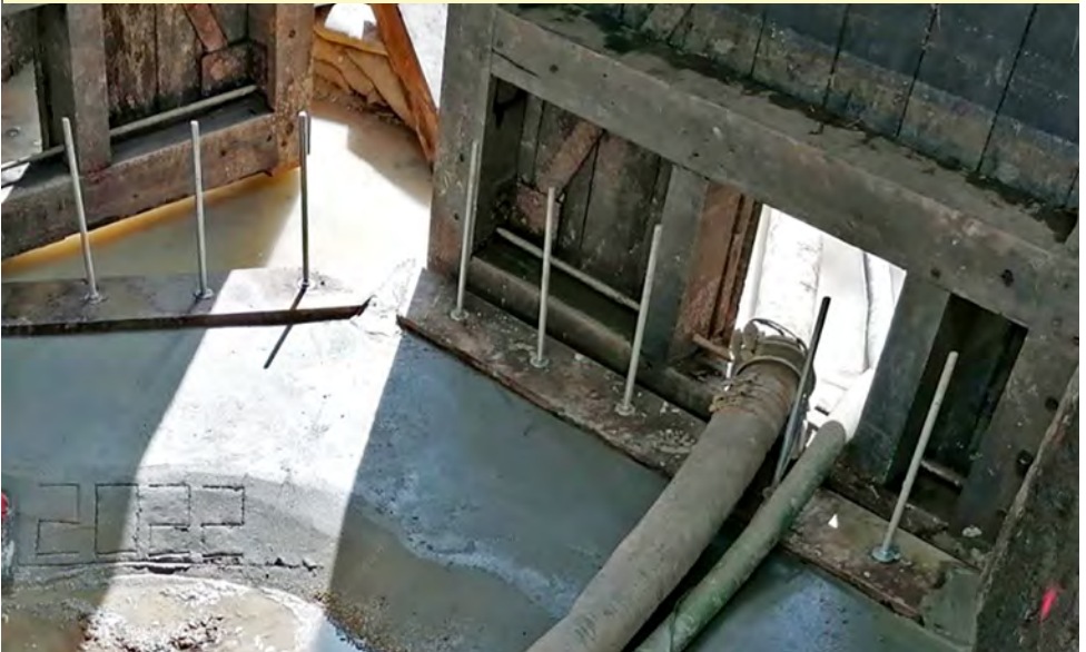
New oak timbers were cut to form new mitres and further reinforced concrete was poured and shaped behind them to complete the construction work. The year was then inscribed in the concrete for posterity.
