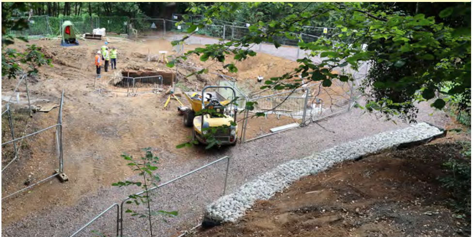
Looking east across the site in mid-August. The bridge site is on the left and looping round to the right the completed bridleway diversion is in place.
