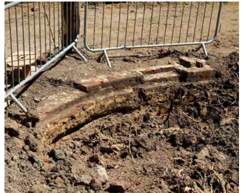
A curved wall on the east side of the Birtley Bridge 2 site was one of the first remains of the original bridge that we uncovered.
