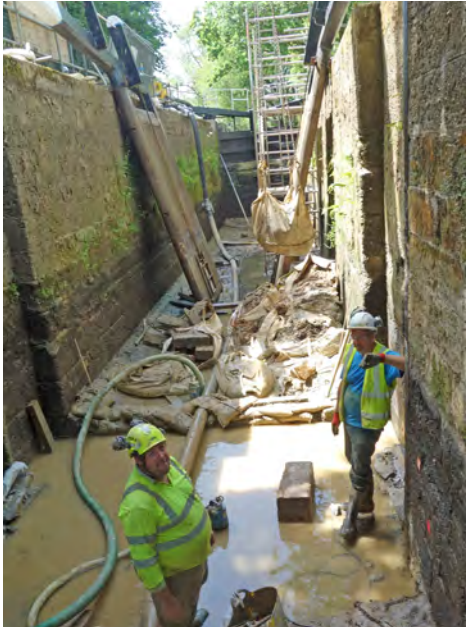
Tonnes of clay and debris had to be removed from the lock by crane.
