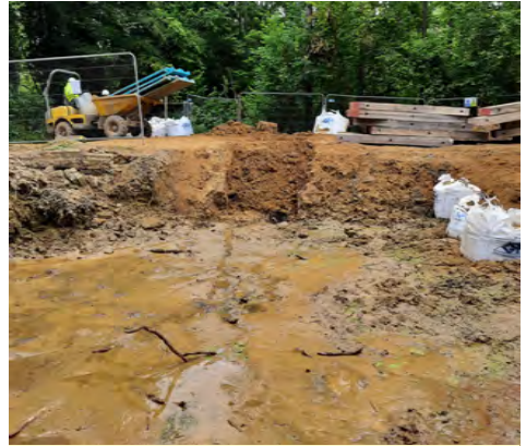
Water flowing into the canal bed from the west bank created a problem.
