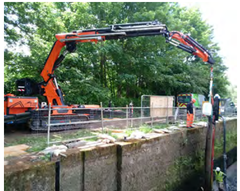
The remedial work required the hiring of a specialist crane to lift out the lock gates and deliver steel bracing props.
