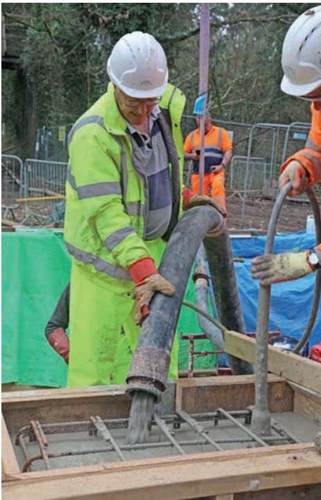
The final concrete pour at Birtley Bridge 2 on March 30th raised the bridge substructure to its final target height.
