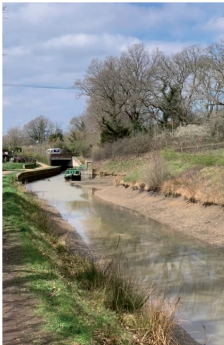
The canal at Loxwood shortly after the criminal damage was discovered, clearly showing the dramatic drop in water level
