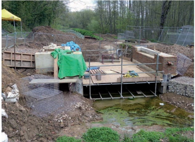
This picture taken in late April shows brick facing on the new Birtley Bridge 2.
