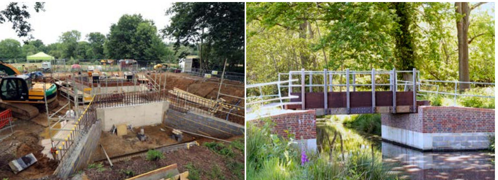
Bridge No 1 – 2019 work in progress, then with finished abutments and temporary bridge deck, 2022
