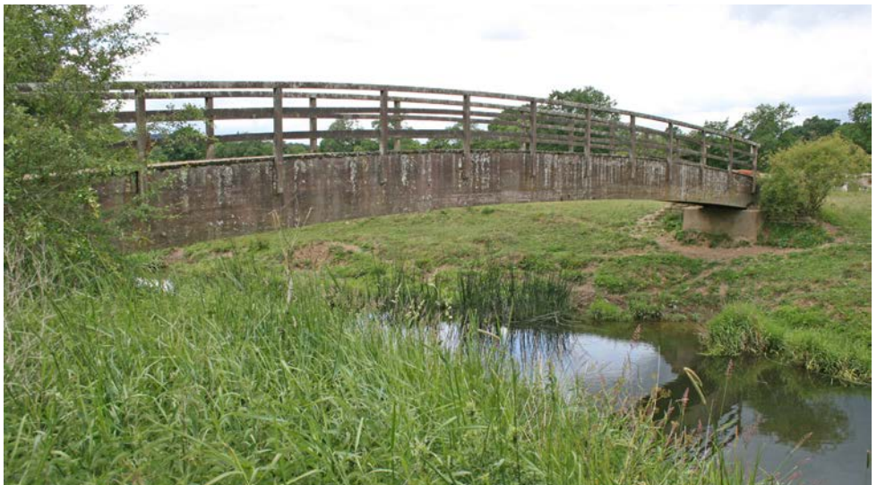
The “Japanese” bridge, a photo taken a few years ago when it was still in use
