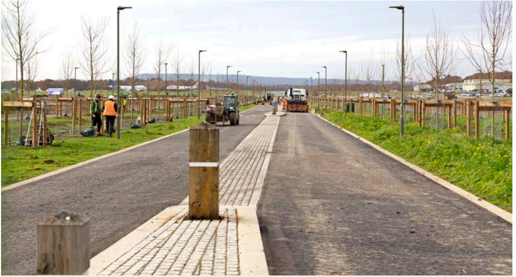
The new eastern access to Dunsfold Park nears completion. In the left distance are two Boeing 747s.
