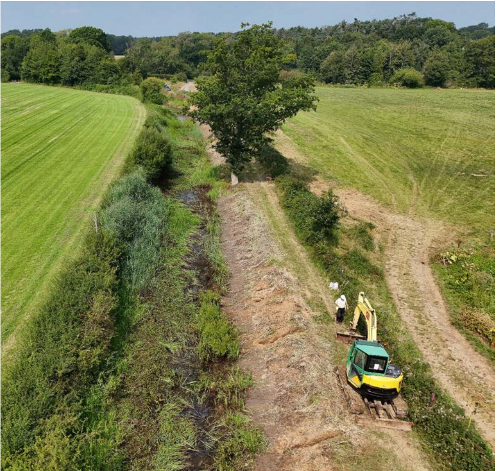
A drone shot of recent bank repair work at Long Meadow. We are looking north – Drungewick Lane is visible in the distance – and the canal is the darker green strip on the left.
