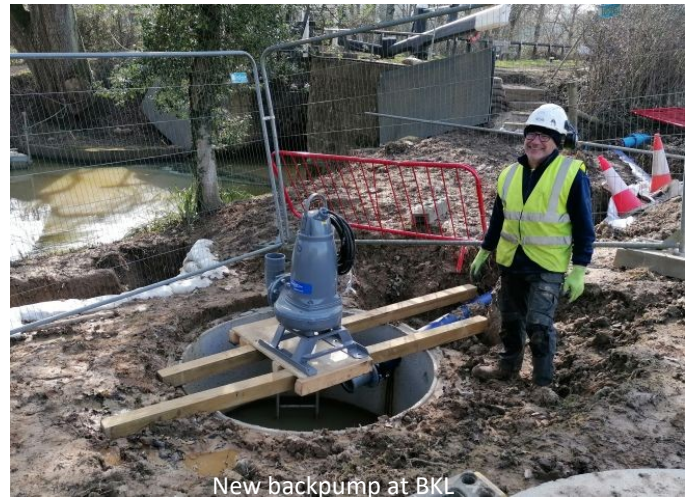
New backpump at BKL
