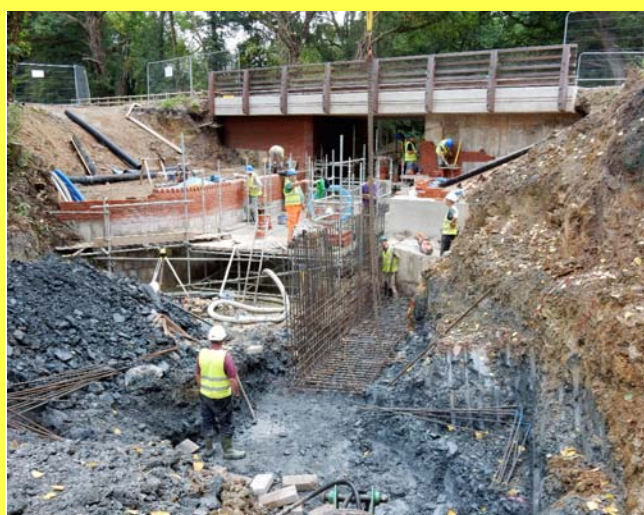
Work at Compasses - still plenty to do before the reopening ceremony (Bill Nicholson)
