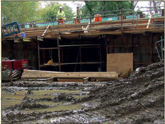
Contractors assembling the steel reinforcement for the concrete deck of the new Compasses Bridge at Alford, one of the Trust's current major projects.
