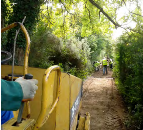
Volunteers upgrading the towpath at Gennets Bridge Lock. They laid around 40 tonnes of type 1 aggregate. (Geoff Thomas)
