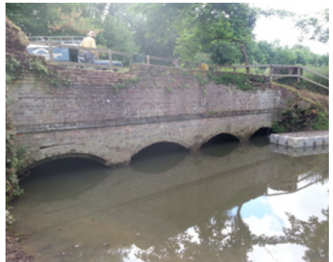
Before, during and after the visit by the Monday Group to shift debris blocking the culverts on the Gosden Aqueduct and clear vegetation from the brickwork. (John Empringham)
