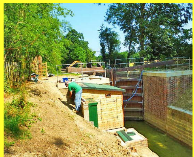
Southland begins to look like a fully functional lock, as the housing for the back pump nears completion in July (Dave Verrall )
