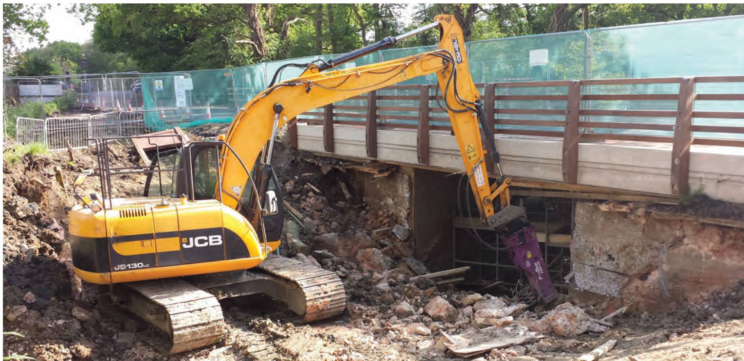
In May 2016, Canal Trust volunteers demolished the causeway that blocked the canal at Compasses in Alford, revealing the timber parapets of the new bridge that has been built immediately alongside.
