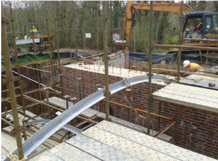
An attractive arched bridge will carry the Sussex Border Path across the canal at Gennets Bridge.
